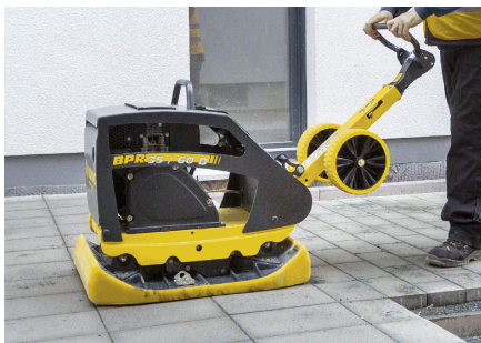
No breakage of paving stones
